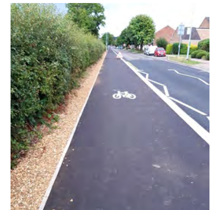
Image 24 - New cycle facilities on Meadway, Leighton Buzzard, part of the Green Wheel inner rim
